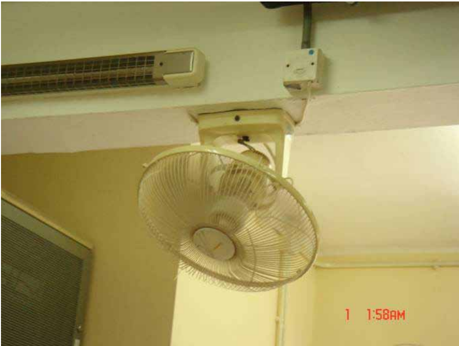
Figure G.2 A ceiling fan for summer cooling and a radiator for winter heating
