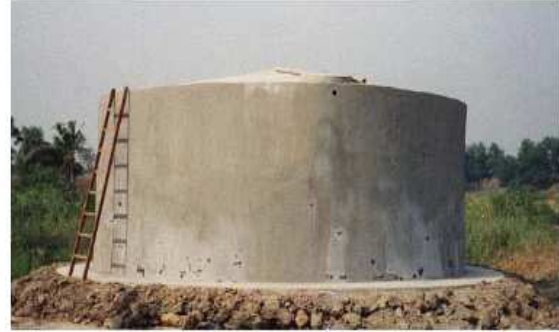
Figure 3. Tank after Two Weeks of Filling
