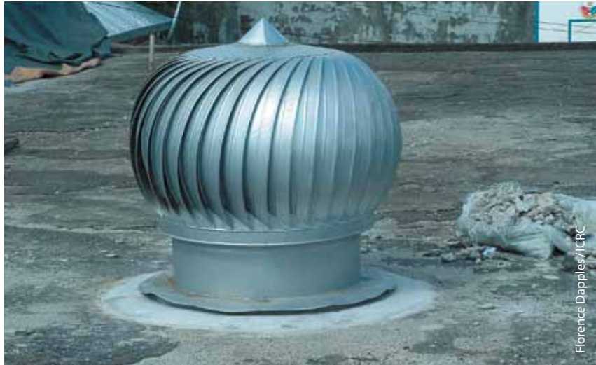
Figure 11 Example of a simple roof ventilation system allowing the evacuation of warm and moist air
