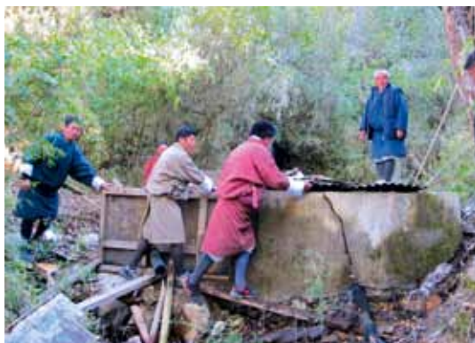
As part of the improvement plan, the damaged wall on an existing intake tank (right) is being repaired, and a supplementary intake tank is under construction (left) in Dhaji, Bhutan
