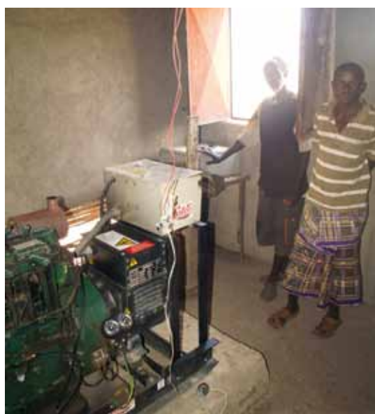
Diesel generator in Magala Adi village, Somali National Regional State, Ethiopia, with caretakers. The village enjoys borehole water from several tapstands at 20 Birr cents a bucket. The next nearest water point is 9 kilometres away, on foot!
