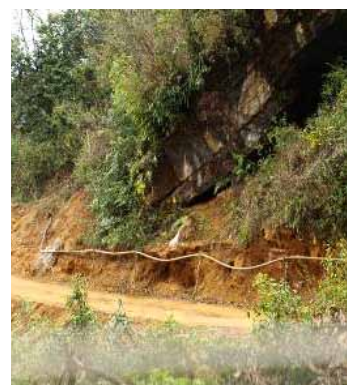
Recent road construction exposed a section of buried mains high-density polyethylene pipeline for a water supply system in Nepal. A vehicle can damage this pipeline (hazardous event), potentially causing disruption of safe water supply to some 70 households (risk).
