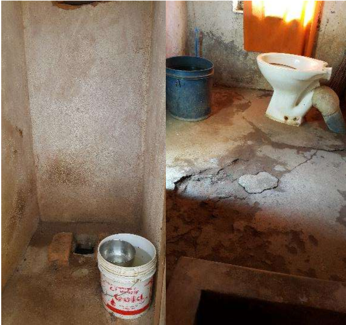
Figure 28: sanitation infrastructure in healthcare facilities with clear concerns for cleanliness and maintenance. Facilities with unimproved forms or even none latrines were also found during the study.
