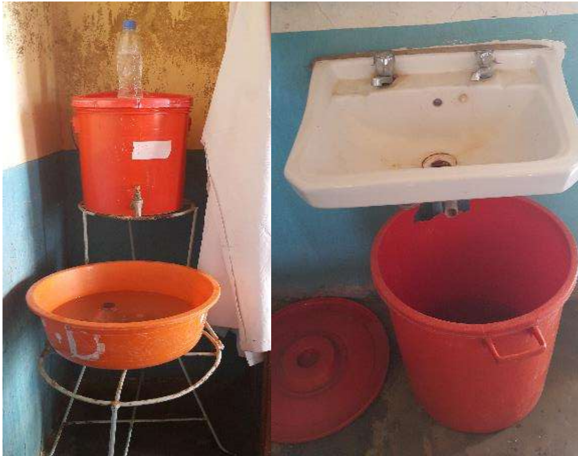
Figure 14: Inadequacy of hand washing infrastructure in HCFs owing to non-adherence to standard provisions and poor operational maintenance. Inappropriate hand washing infrastructure is also associated with poor drainage of contaminated waste water.
